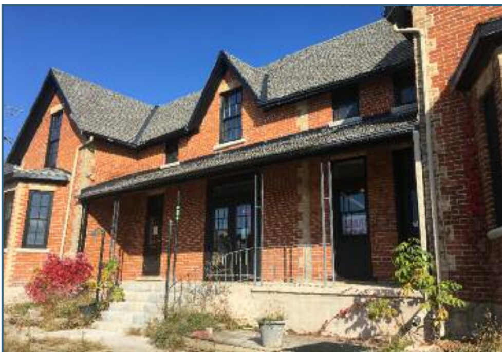
Removing the paint from the front façade of 219-221 Hurontario Street (known as the Olde Town Terrace) revealed the beauty of the signature Collingwood brickwork.
